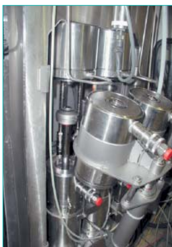
Open for cleaning, inspection and maintenance
